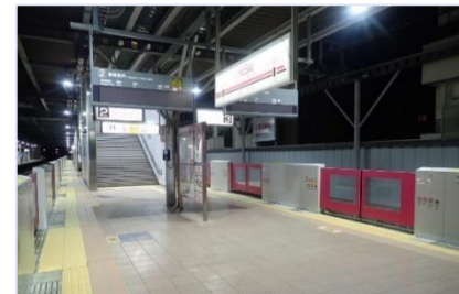
Installation of sliding doors on platform No. 3 at Tobitakyu Station, which is closest station to venue
