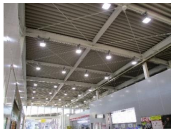
LED lighting installed inside stations (Plan to install in Eifukucho Station and other stations in FY2023)
