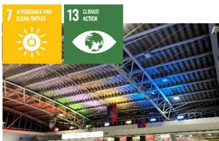
《Switch to LED lighting》
