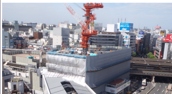
Both demolition and new construction work are proceeding in parallel (photo taken in August, 2012)
